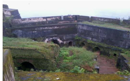
Figure 11: Dampness in the vicinity of Fort.
