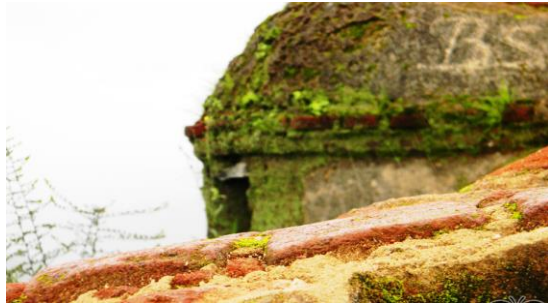
Figure 8: Damage due to Wind and Graffiti.
