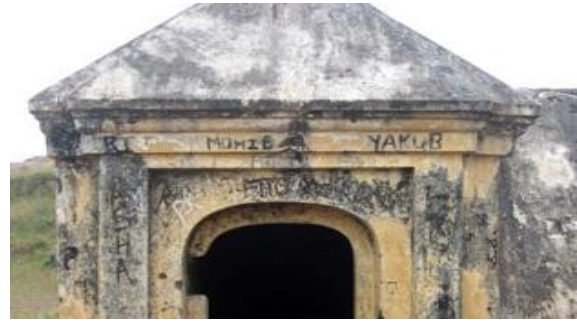
Figure 9: Graffiti and defacing of the walls.
