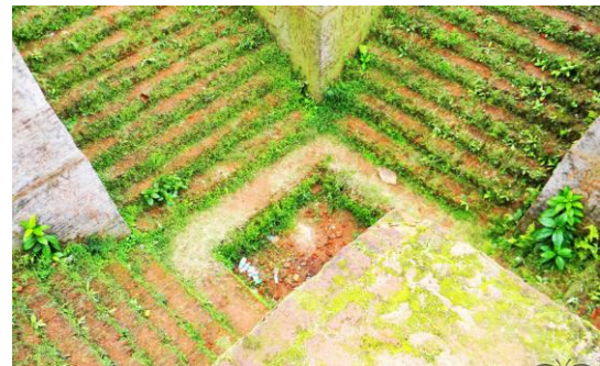
Figure 5: Vegetation on Fort's internal surfaces.
