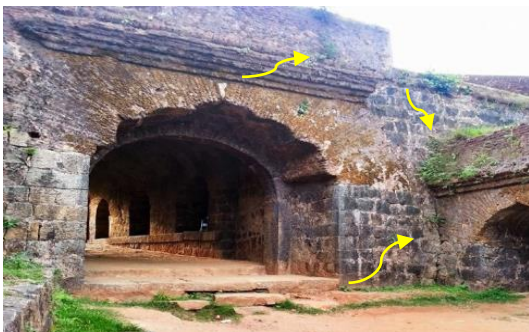
Figure 6: Vegetation growth in crevices/gaps.
