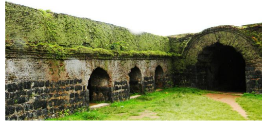
Figure 3: Vegetation growth on the wall.
