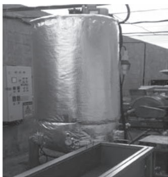
Figure 9. Insulated AN solution tank reservoir.
