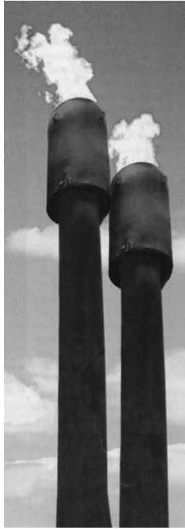
FIGURE 10.4 Elevated open candlestick flare with windscreen.
